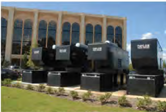
Photo: Taylor Power Systems Each TD350 handles one story of the building.
